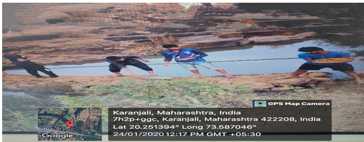
Conservation of Rain water Harvesting, Vanrai Bandhara was build nearby river of Devgoan. 24/01/2020
