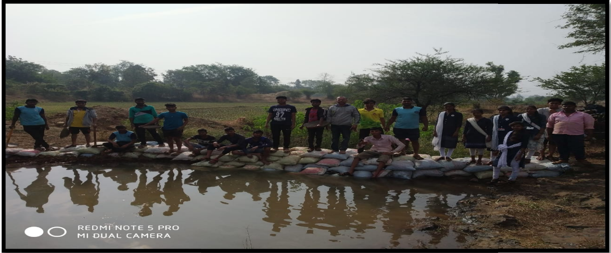
Conservation of Rain water Harvesting, VanraiBandhara was build nearby river of Devgoan. 19 December 2019
