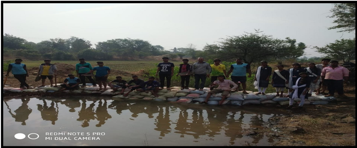
Conservation of Rain water Harvesting, VanraiBandhara was build nearby river of Devgoan. 19 December 2019
