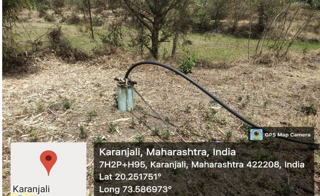
Photo No.3.1 Shows Borewell used for water supply.
